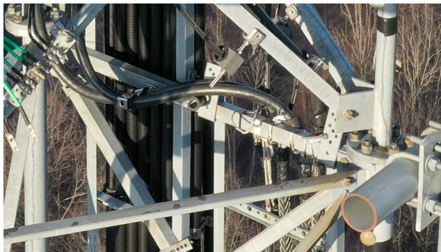
Figure 2 - Steel angle is flexing due to weight and cable and grip installation method.
