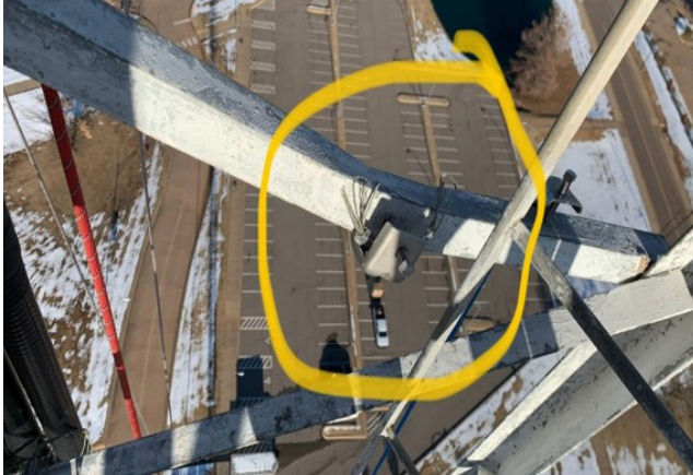
Figure 1 - Failed bracing due to improper WMG attachment.
