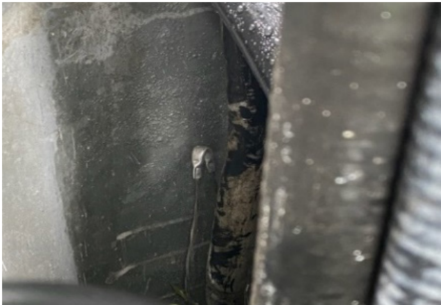
Figure 4- Failed J-hook from weight of hybrid cable on monopole.
